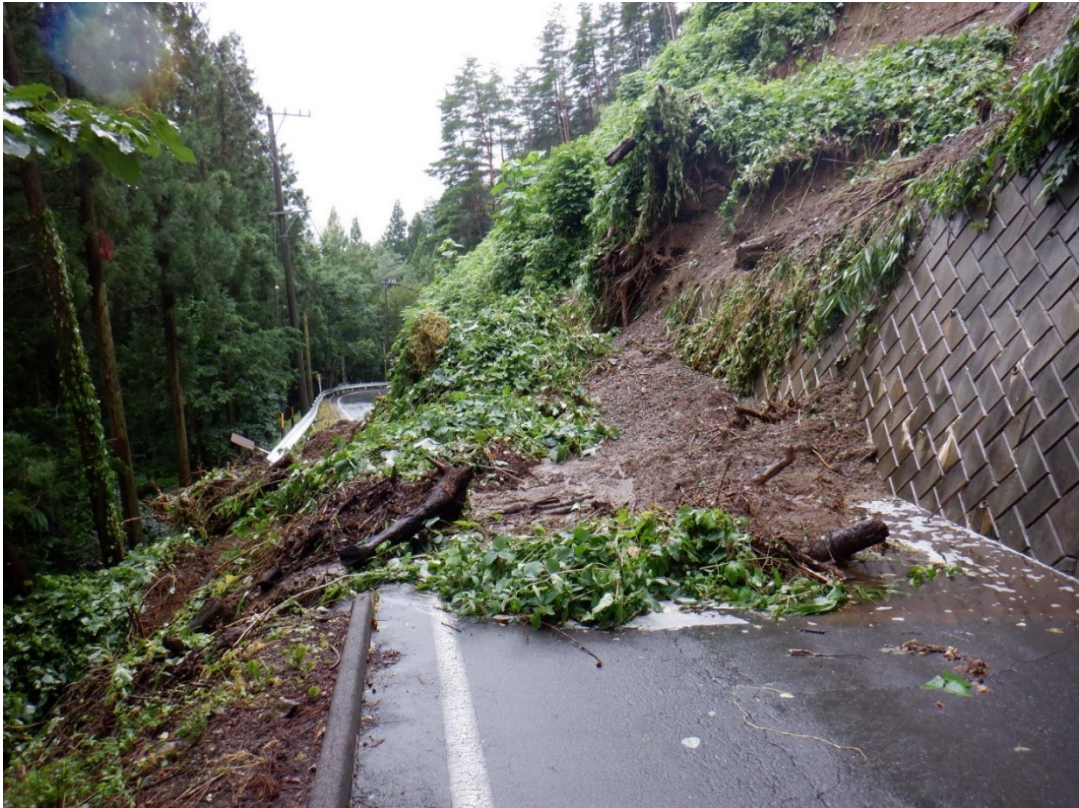
Heavy rain disaster of August 14 th - 15 th , 2021
